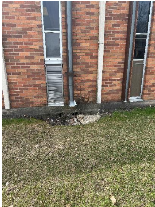
Erosion and undermining beneath downspout.
