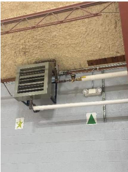
Operational Unit heater serving Gym
