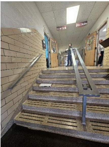
Non-compliant handrail extension
