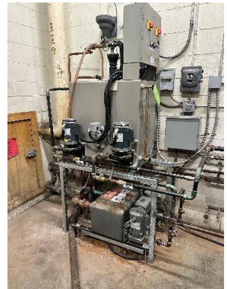
Steam Condensate collection/pumps
