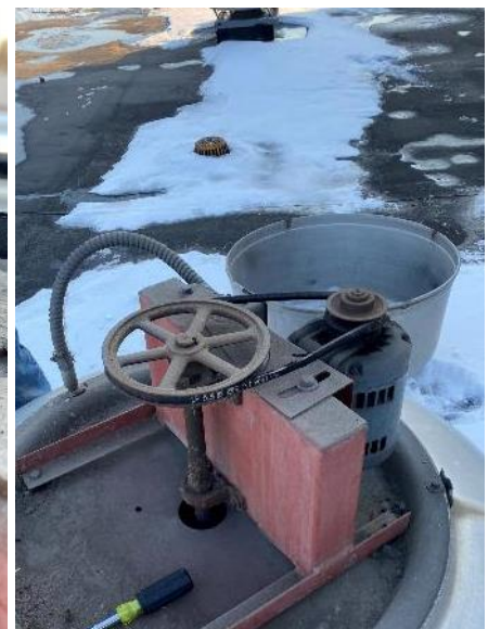
PRV – Maintenance Required
