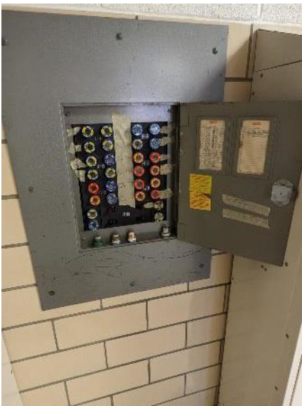
Panel in Corridor outside Classroom 5W
