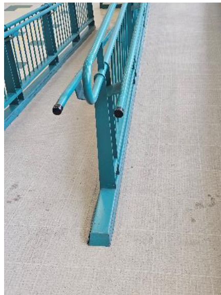
Non-compliant handrail extension
