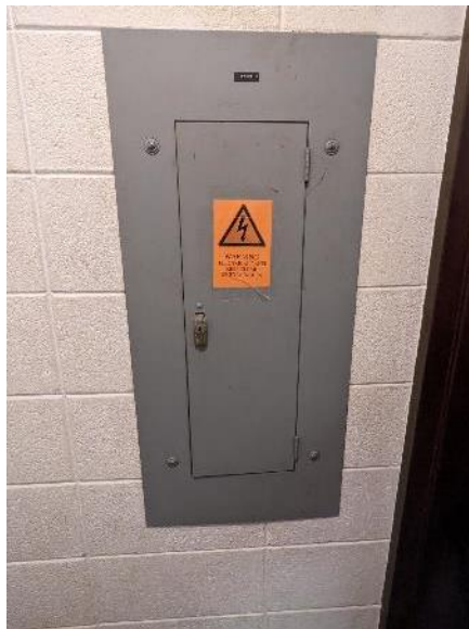
Panel F in Janitor's Closet A119
