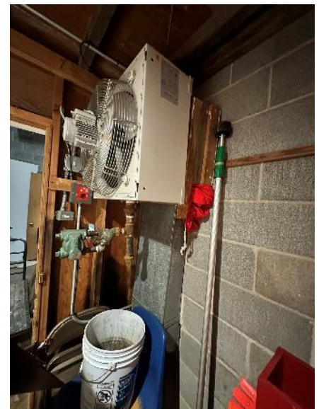
Disconnected Unit Heater
