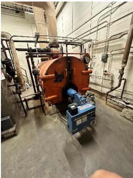
Fuel Oil Boiler
