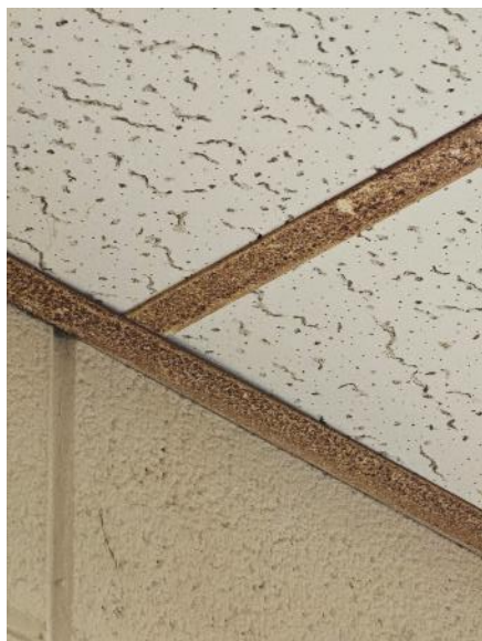
Rusted ceiling grid
