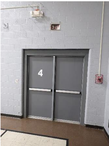
Damaged Exit Sign in Gymnasium 162
