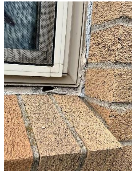
Deteriorated window sealant
