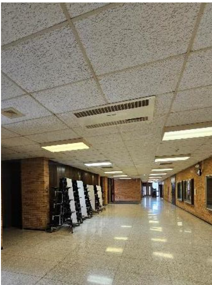
Recessed Ceiling Heater - Lobby
