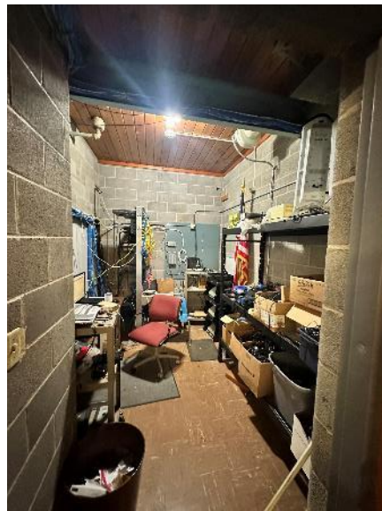
IT room with inline fan in upper right
