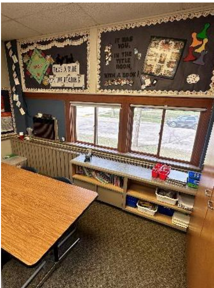
Through wall AC unit
