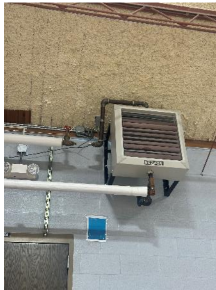
Disconnected Unit Heater
