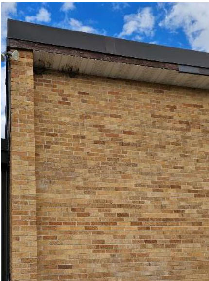
Missing section of metal fascia
