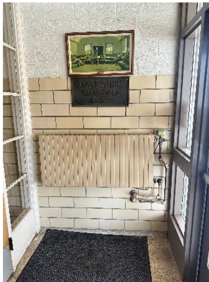
Vestibule Steam Radiator
