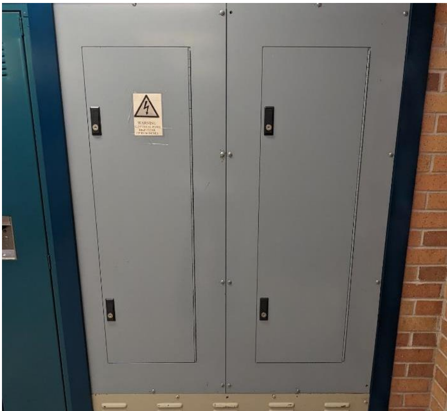
Double-tub Panel in Corridor 136A outside Classroom ECFE 5E
