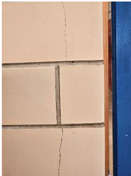
Cracking at wall tile
