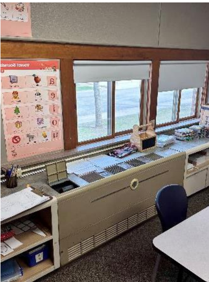
Classroom Unit Steam Ventilator
