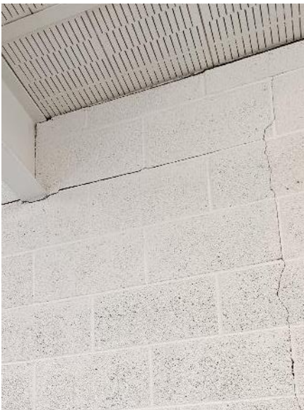
Wall cracks – likely due to settlement forces
