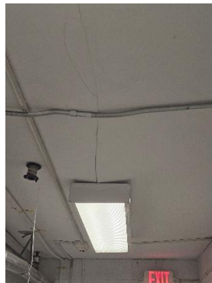
Cracked and sagging ceiling near Kitchen
