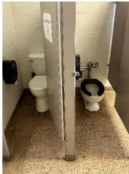
Replacement water closets do not match
