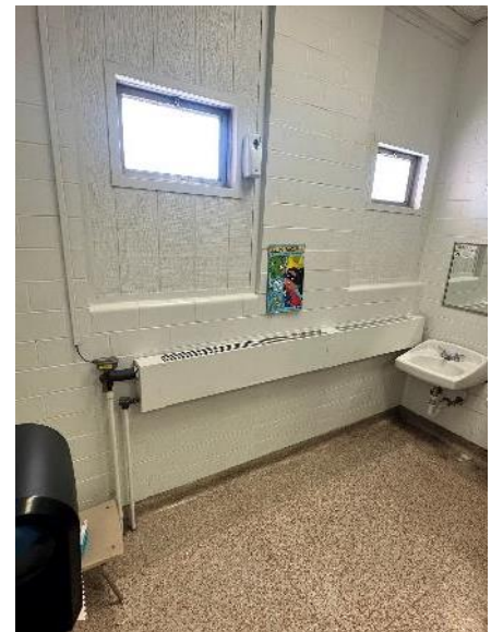
Restroom Steam Radiator
