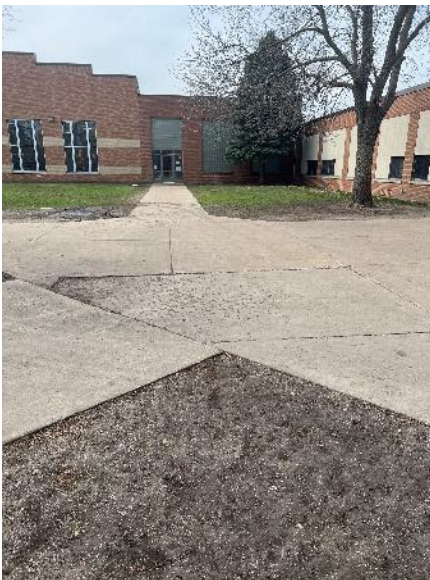
Drainage issues in green space.
