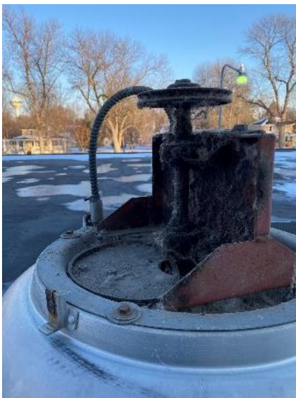
PRV – Missing motor.
