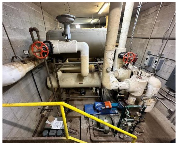
Steam to Hot Water Distribution / Pumps
