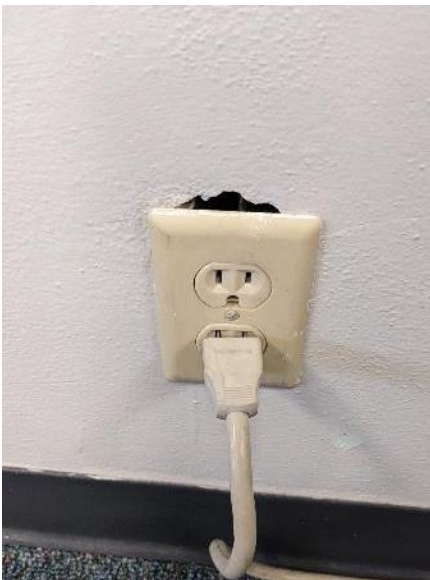
Receptacle in Kindergarten 17W
