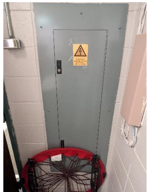
Panel in Office Area Adjacent SPED 8E
