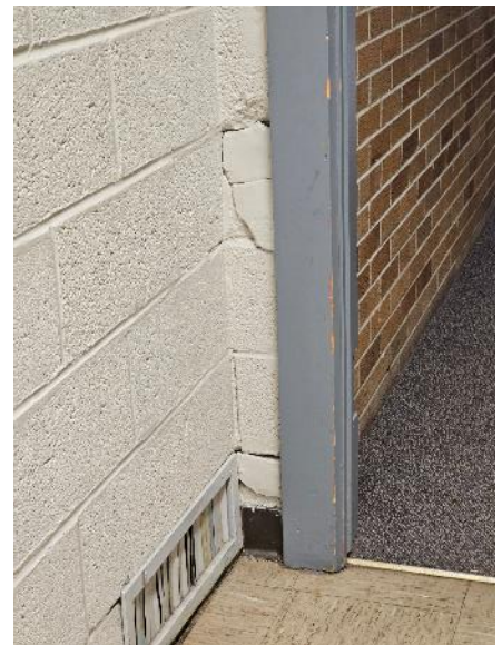
Cracking near interior hallway opening
