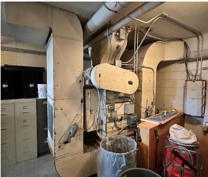
Indoor AHU – Heating Only
