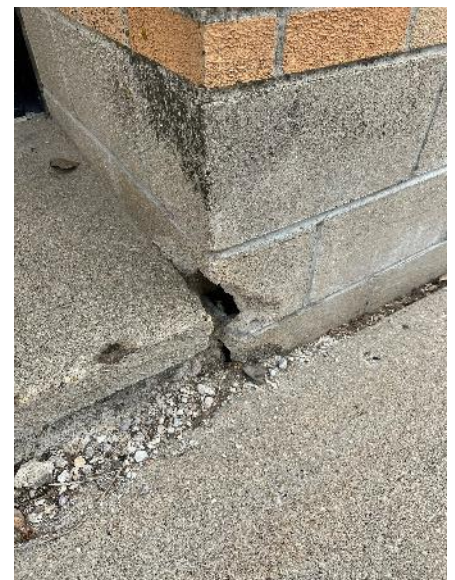
Damaged corner brick
