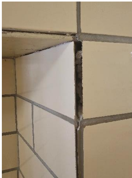
Damaged wall tile grout
