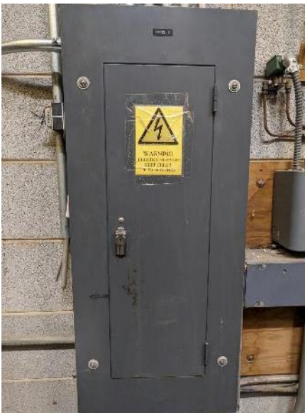
Panel E in Boiler Room A133
