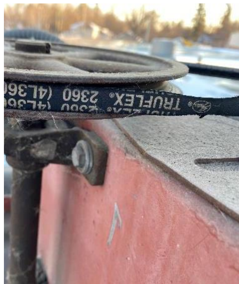
PRV – Maintenance Required
