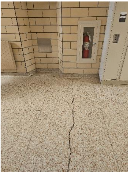
Cracking across hallway
