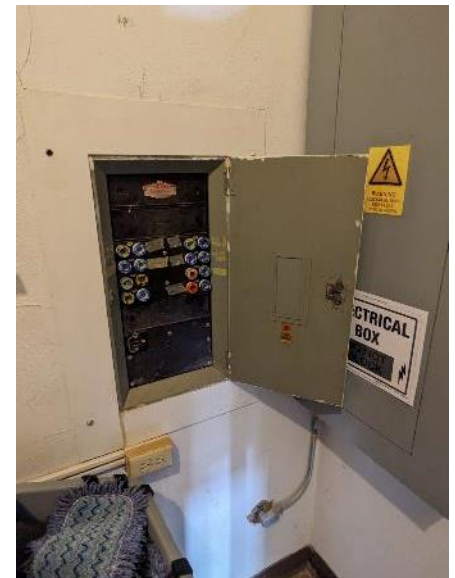
Panel in IT/Janitor's Closet adjacent Rm 17W
