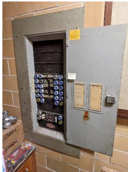
Panel in Janitor's Closet across from Rm 9W
