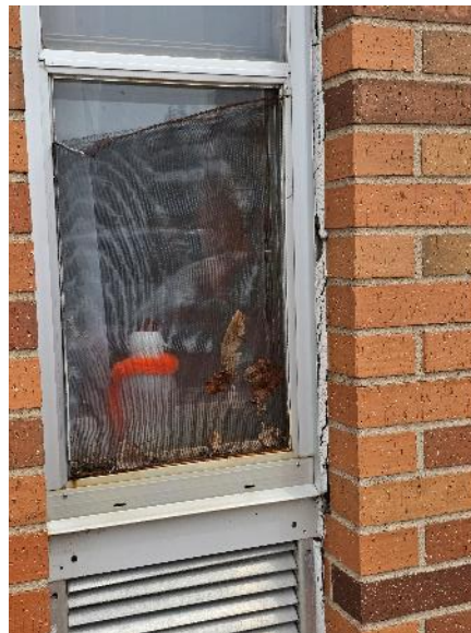
Deteriorated window sealant
