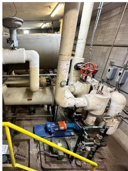
Steam to Hot Water Exchanger
