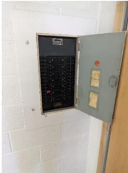
Panel in Hallway outside Gymnasium 162
