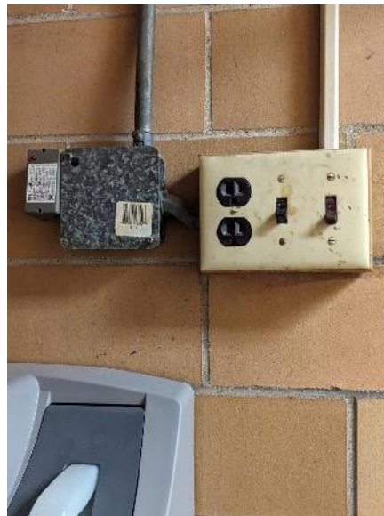
Non-GFCI Receptacle in Janitor's Closet
