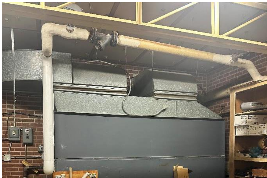
Steam distribution piping to AHU
