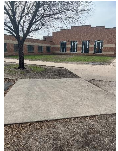
Drainage issues in green space.
