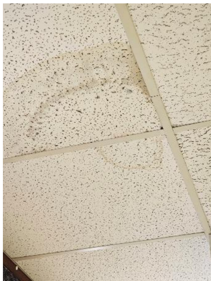
Stained ceiling tile
