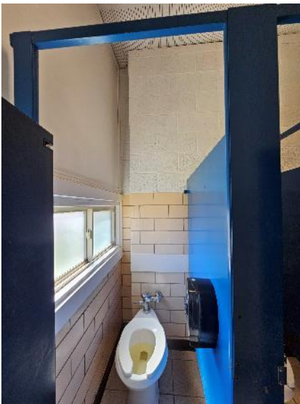
Stalls lack compliant floor space & grab bars
