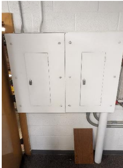
Two Panels located in Custodial Office/Storage 117
