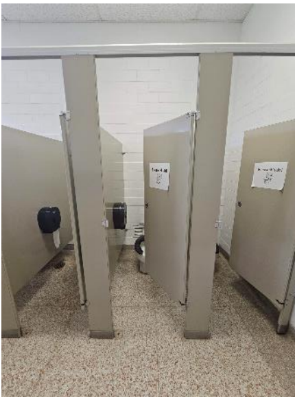
Stalls lack compliant floor space & grab bars
