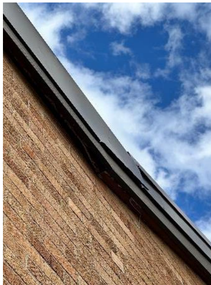
Wood rot at sub-fascia
