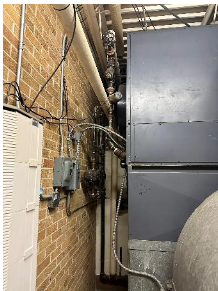
Steam distribution piping to AHU
